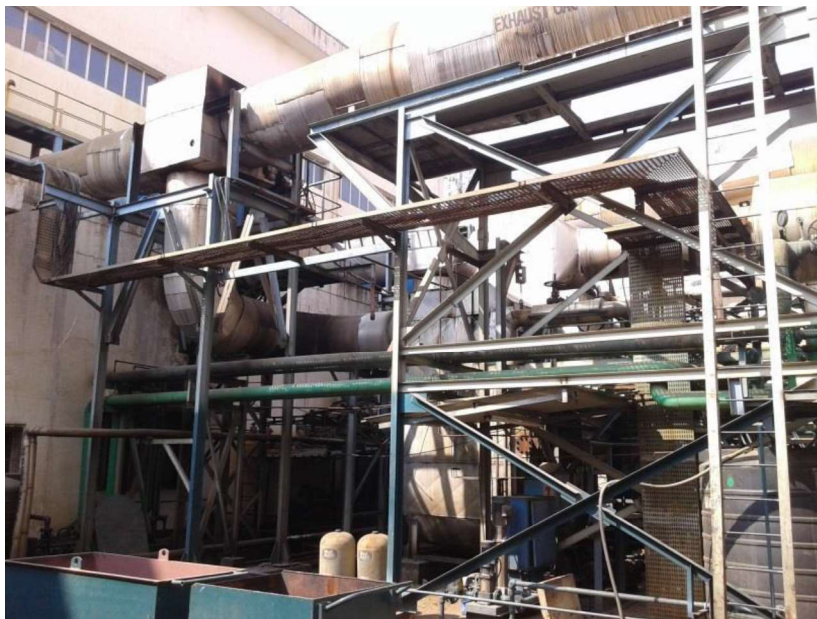
Picture 19 – HRU Unit
