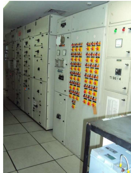
Picture 22 - Battery charger panel.
