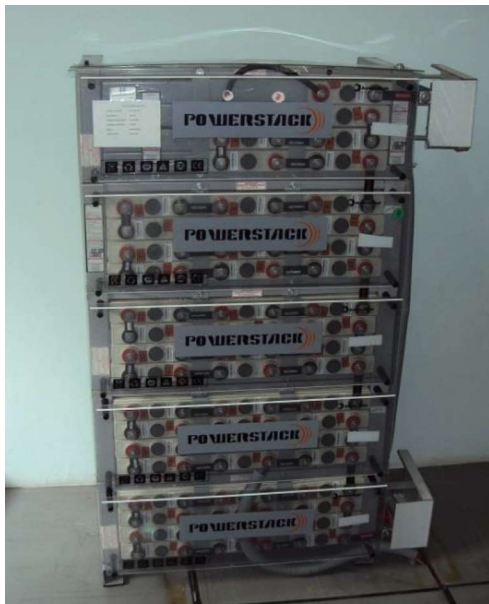
Picture 21 – Battery Bank
