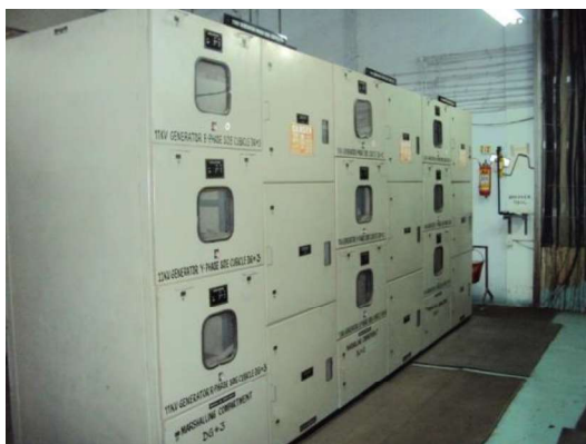
Picture 25 – 11 KV Generator phase side
