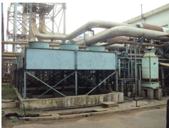
Picture 3 (Radiators – DG 1)
