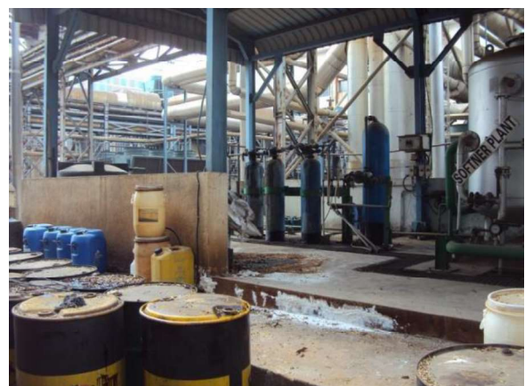
Picture 16 – DM Water plant.
