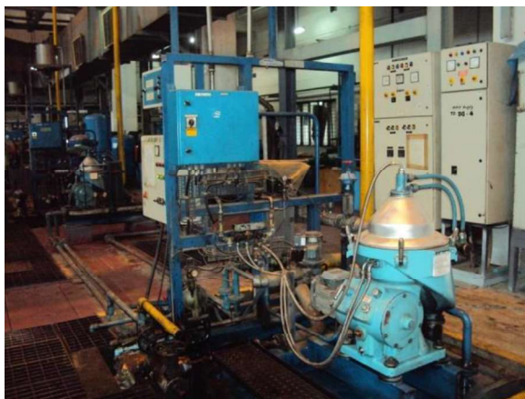
Picture 4 (DG – 3 Lube oil separator.)
