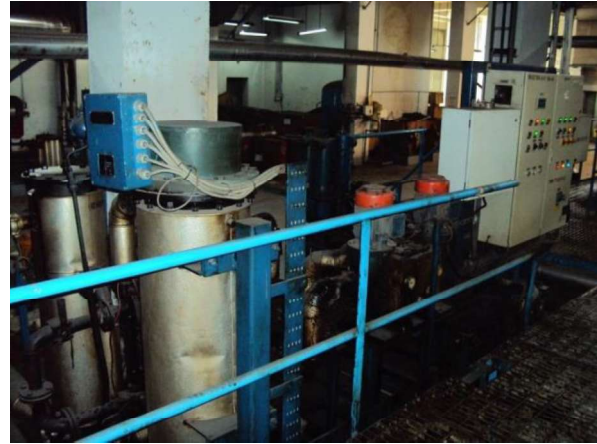
Picture 8 – DG – 5 Fuel Booster unit.
