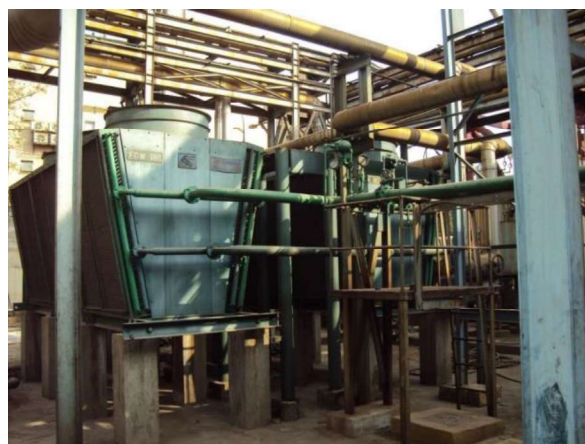
Picture 6 (DG – 4 Radiator unit.)
