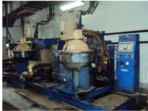
Picture 10 - DG – 5 HFO Separators.
