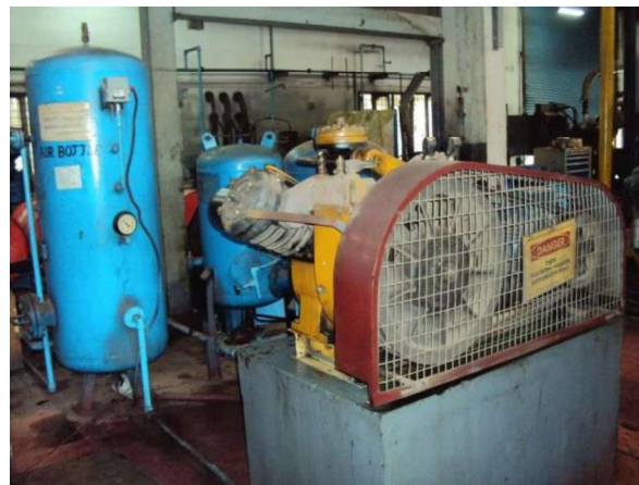
Picture 14 – Air compressors
