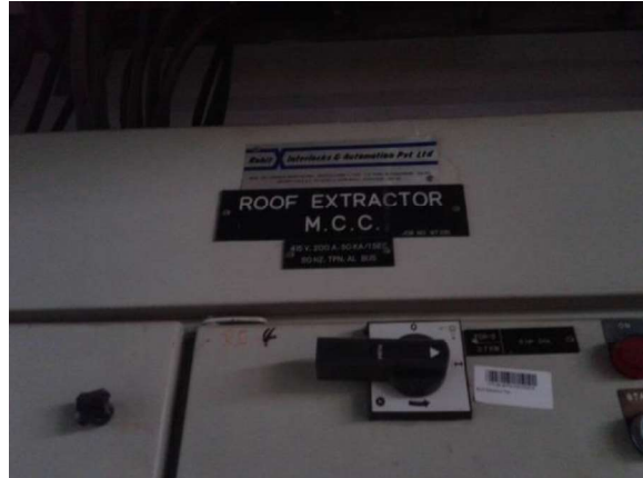
Picture 18 – MCC panel of Ventilation System
