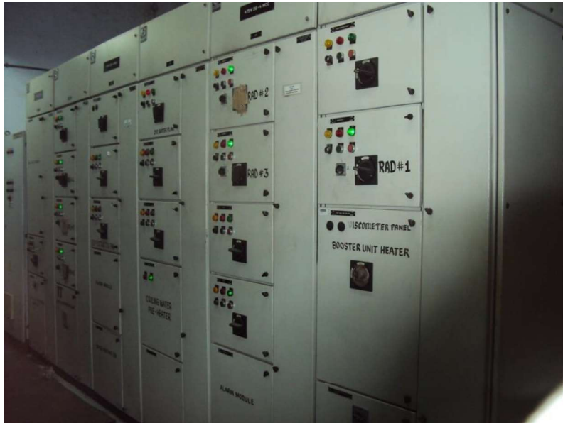
Picture 24 – MCC panel
