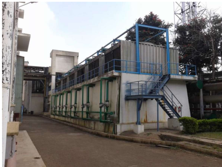
Picture 29 – Cooling Tower
