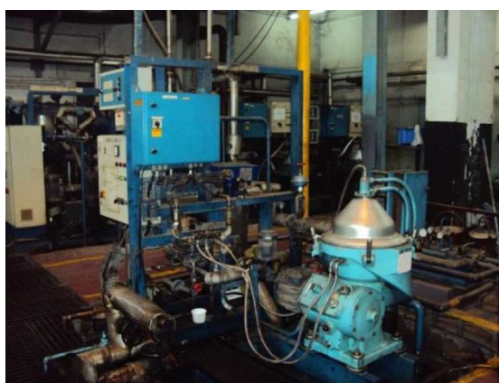
Picture 2 (Lube Oil Separator – DG 1)
