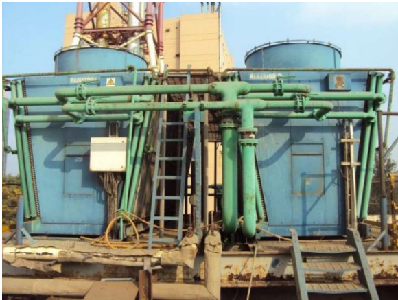
Picture 9 - Radiator Unit (DG 5)
