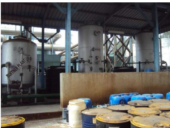
Picture 15 – Water softener plant.
